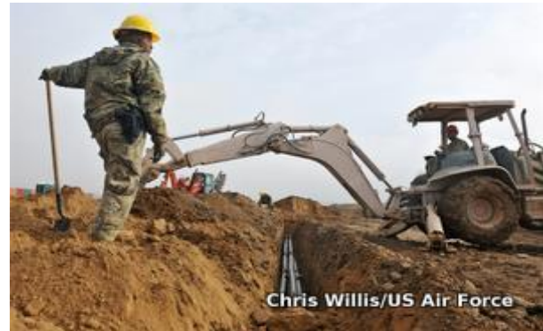
Figure: Fiber-optic networks are expensive to construct (largely because it costs so much to dig up streets). Because the labor and construction costs are much more expensive than the cable itself, many network operators deliberately lay much more cable than they currently need. (Ref. Picture by Chris Willis courtesy of US Air Force)
